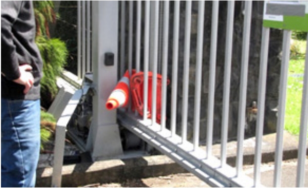
FIGURE 3: The gate, closed, with cone caught in gate housing
