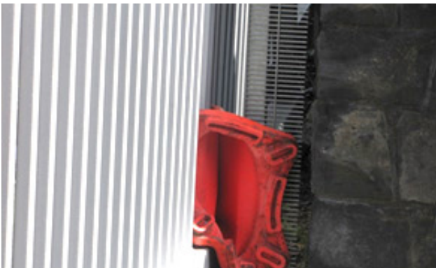
FIGURE 4: The fully closed gate showing cone from the side the child was playing on
