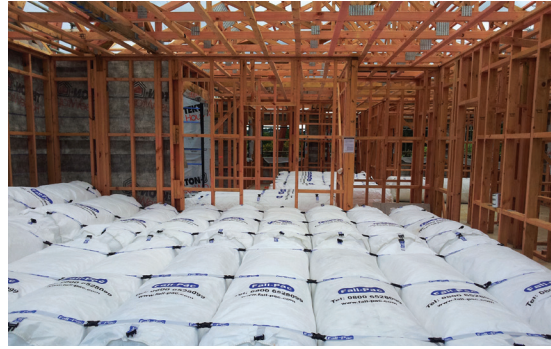
Figure 4: Bean bags being used as a fall mitigation measure during roof work (Image courtesy of Fall-Pac NZ Limited).
