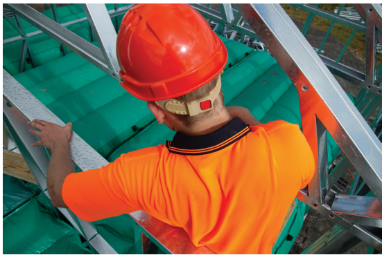
Figure 3: Air bags being used as a fall mitigation measure during roof work (Image courtesy of Airtek Safety Products Ltd).
