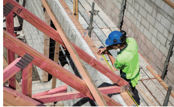
Figure 6: Measuring and installing purlins from an external work platform (Image courtesy of Site Safe New Zealand Inc).
