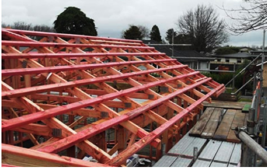
Figure 5: A safe working platform was used at the start of the sequential installation of the purlins/roofing battens.
