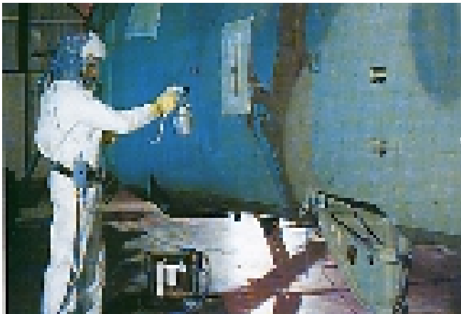
Spray painting exposes an operator to mists and vapours.
